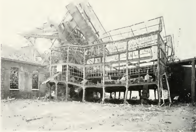
COAL-PIT AND SCREENING INSTALLATION AT DROCOURT, DESTROYED WITH EXPLOSIVES BY THE GERMANS.
