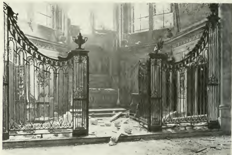
CHAPEL OF ST. JOHN THE BAPTIST DAMAGED BY SHELL (left-hand side of Apse).
