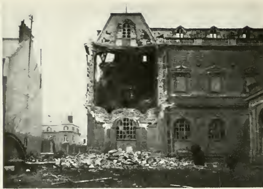
MUSEUM — RIGHT WING OF REAR FAÇADE DAMAGED BY AERIAL TORPEDO IN 1918
