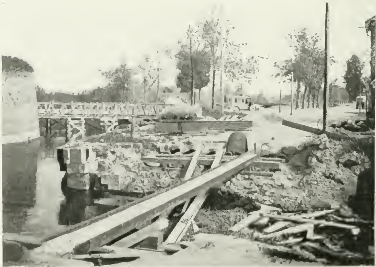
THE OLD RAMPARTS IN THE FAUBOURG DE PARIS. In the foreground: The destroyed bridge; In the background: The temporary bridge; On the right: The N. 17 going towards Villers-Carbonnel.
