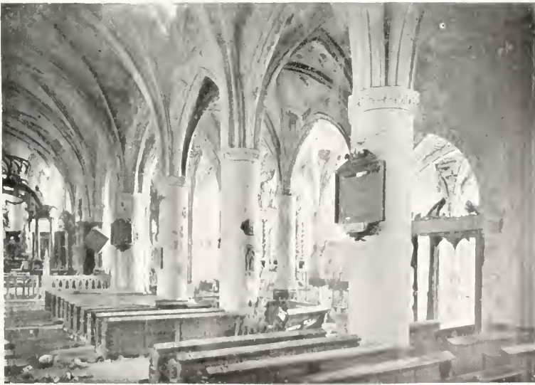
DUN-SUR-MEUSE. DAMAGED NAVE AND SOUTH AISLE OF CHURCH (SEEN FROM THE CHOIR)
