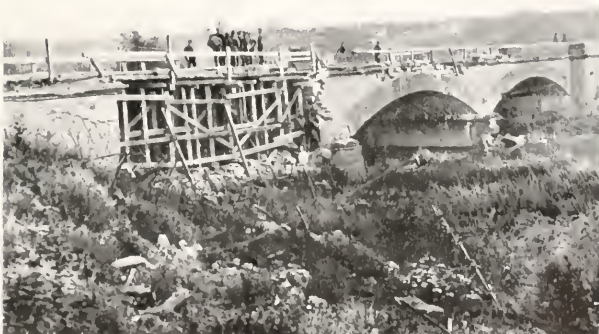
BOUREUILLES. THE 27TH ENGINEERS REPAIRED THIS BRIDGE OVER THE AIRE IN AN HOUR AND A HALF (N. 46 crosses the bridge.)
